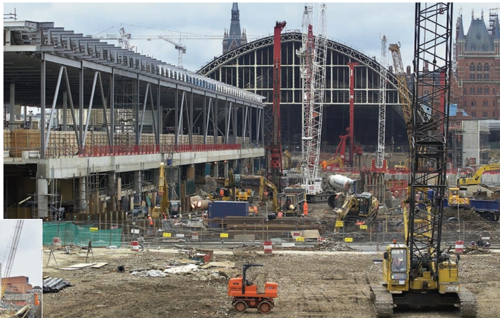
View looking toward the St. Pancras Station shows work on the Thameslink Box and half the deck extension.
